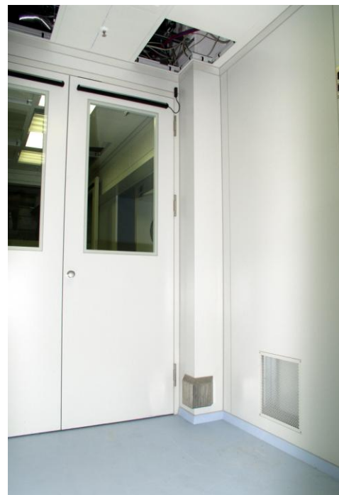
equipped with fenders and ventilation
